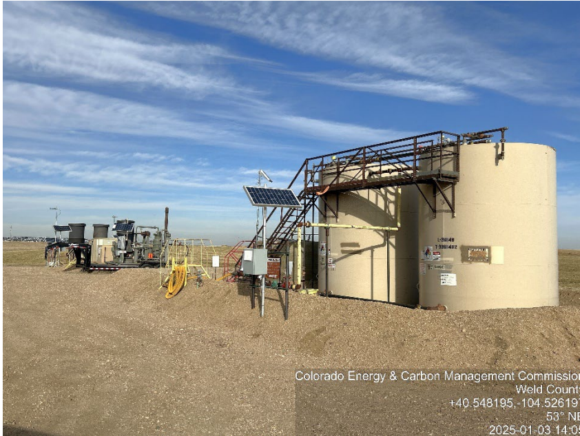
Photo #3 Wilson 4-26, 3-26 Battery site Inactive | Shut-down
