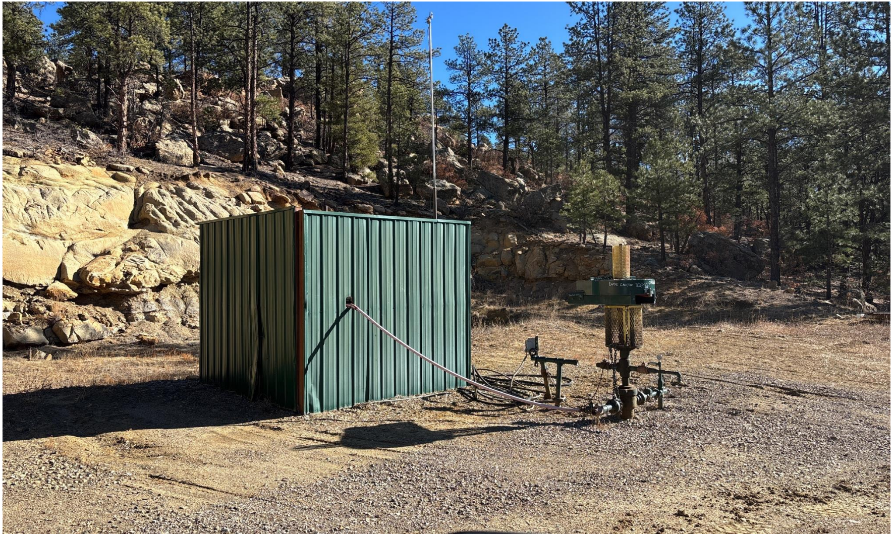
PHOTO 3: ORIG. WELLHEAD AND EQUIPMENT.
