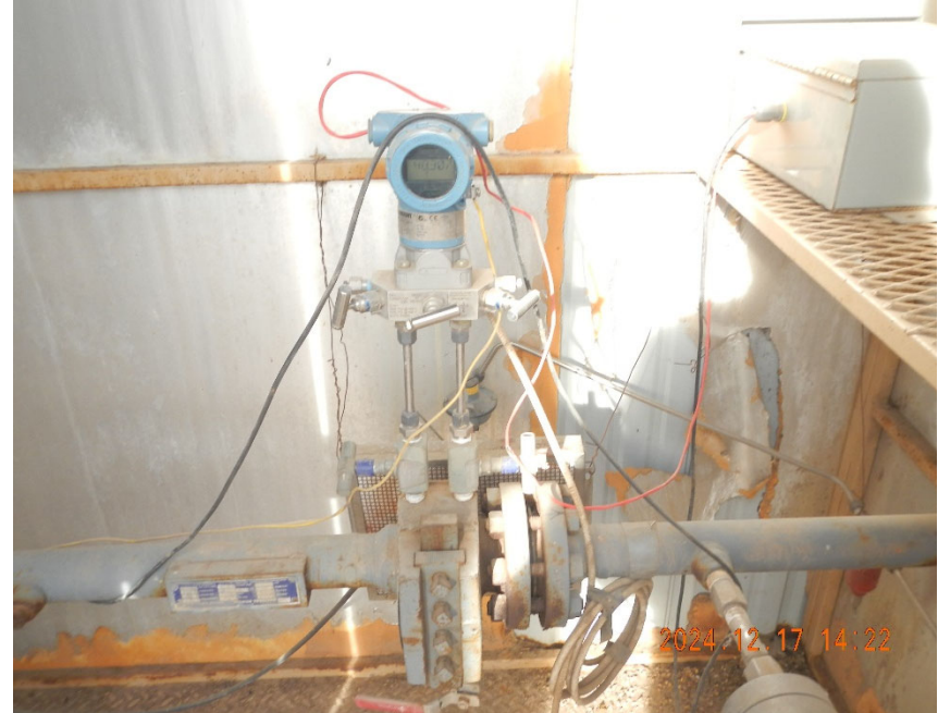
4. Gas meter inside meter shed.
