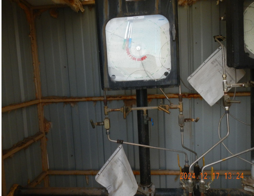
5. Gas meter inside meter shed.
