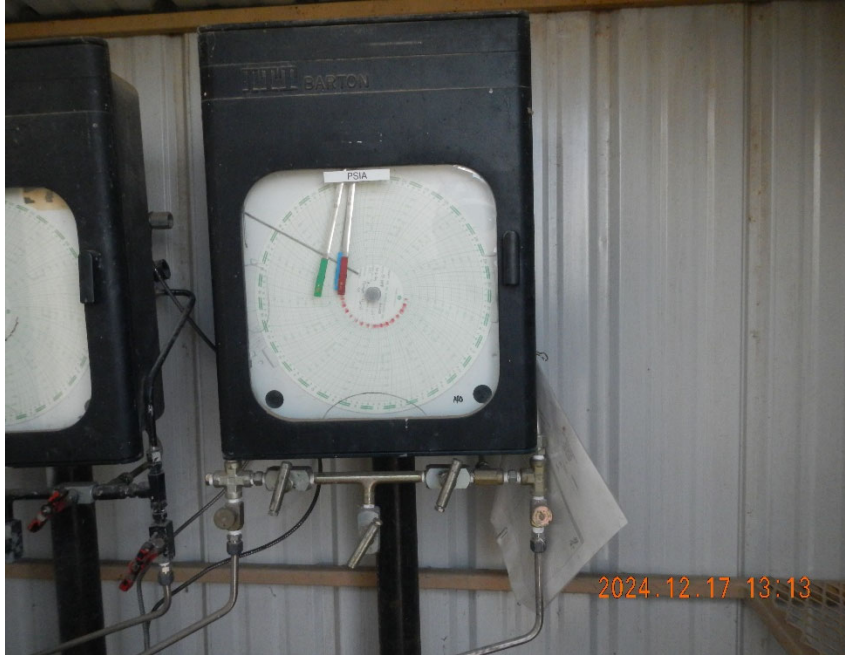
5. Gas meter inside meter shed.
