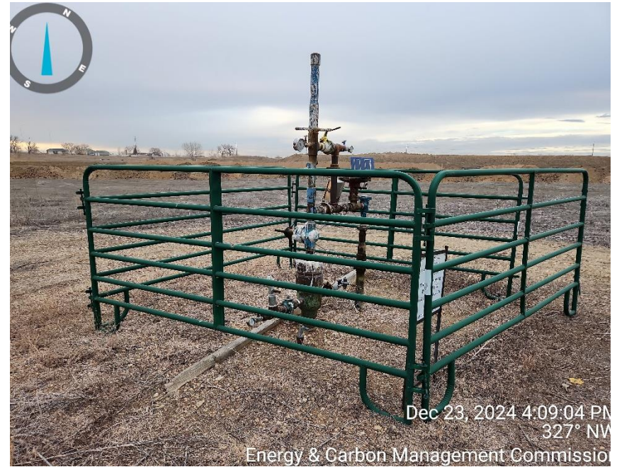
Photo 2 well head and equipment
