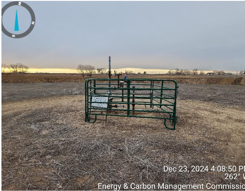
Photo 1 well head and equipment
