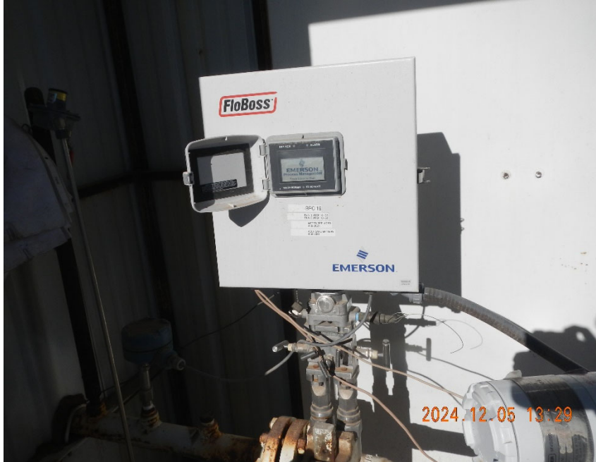
5. Gas meter inside shared meter shed.
