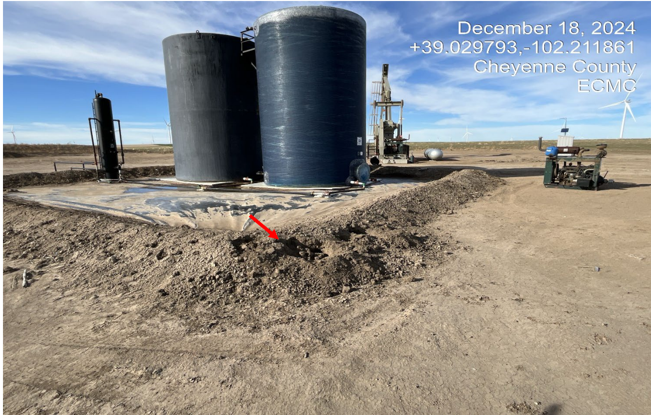
Photo 4. There are animal burrows in the side of the berm. The earthen berm is not designed to resist degradation from erosion.
