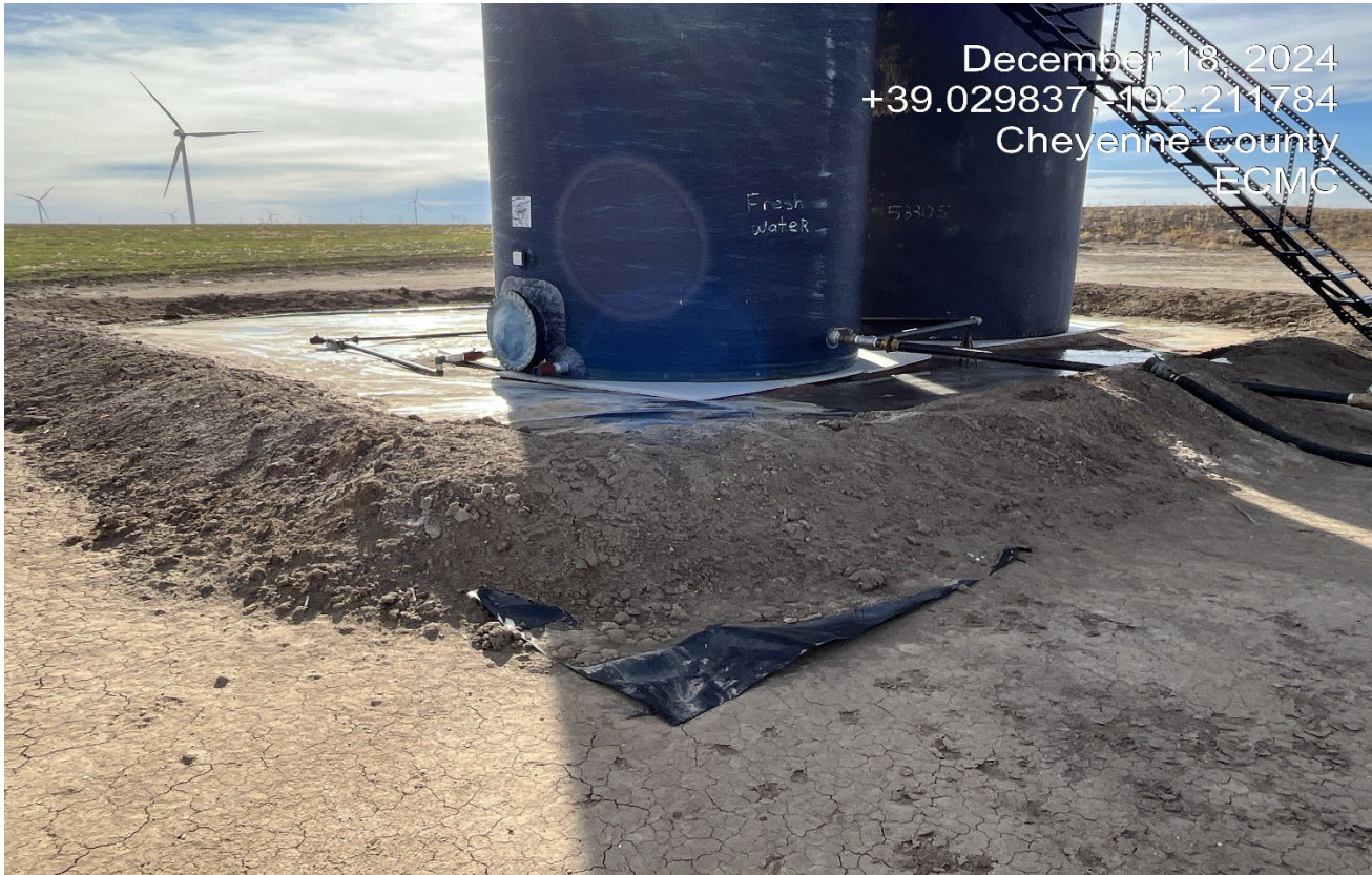
Photo 3. Facing toward the tank battery. The earthen berm is not designed to resist degradation from erosion.
