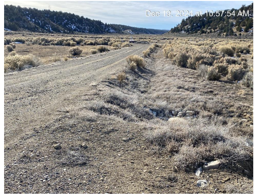
Well pad from Southwest corner of production pad
