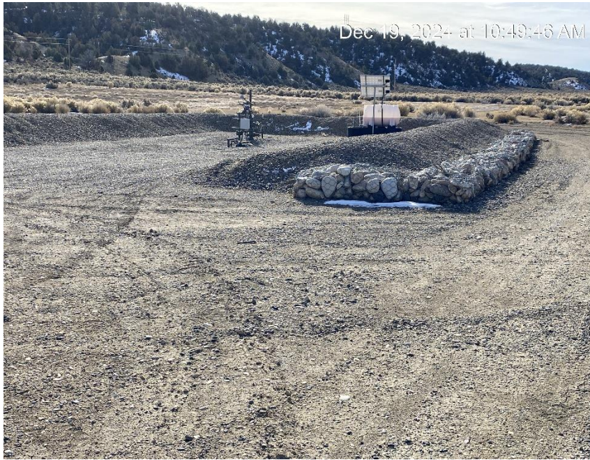
Well pad from Northeast corner
