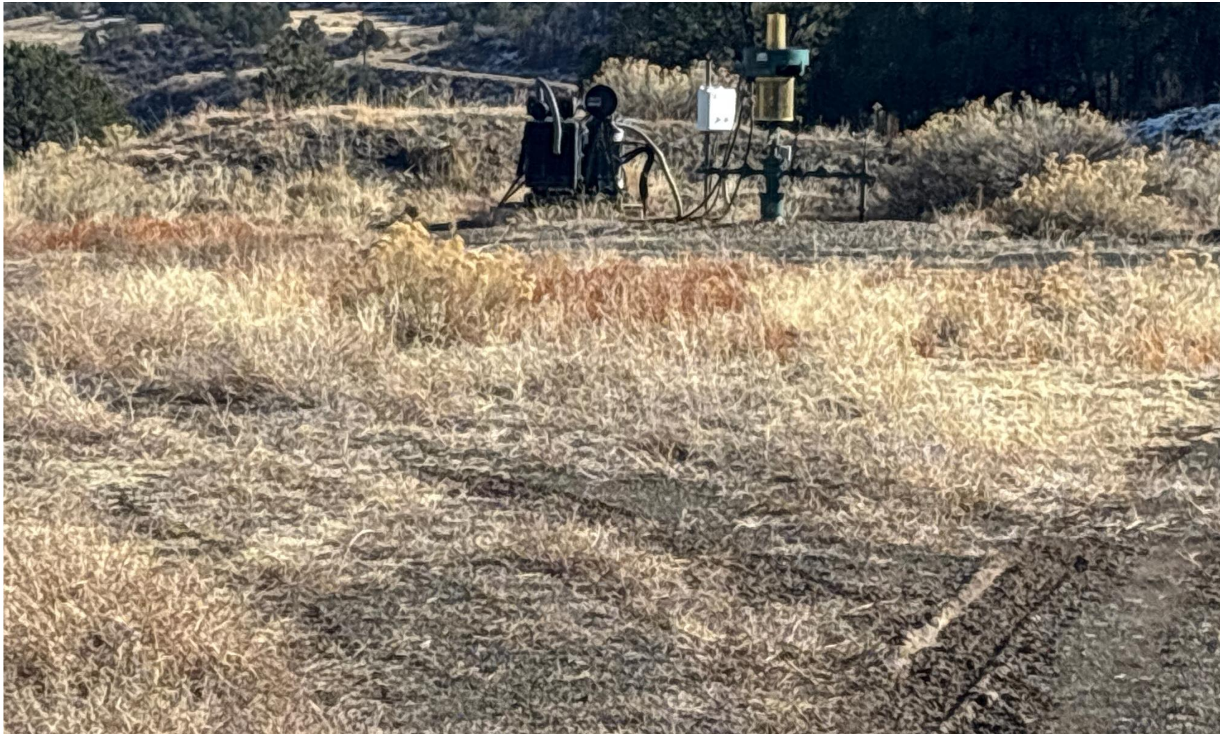
PHOTO 4: WEEDS NEED MAINTAINED AROUND EQUIPMENT AND LOCATION.
