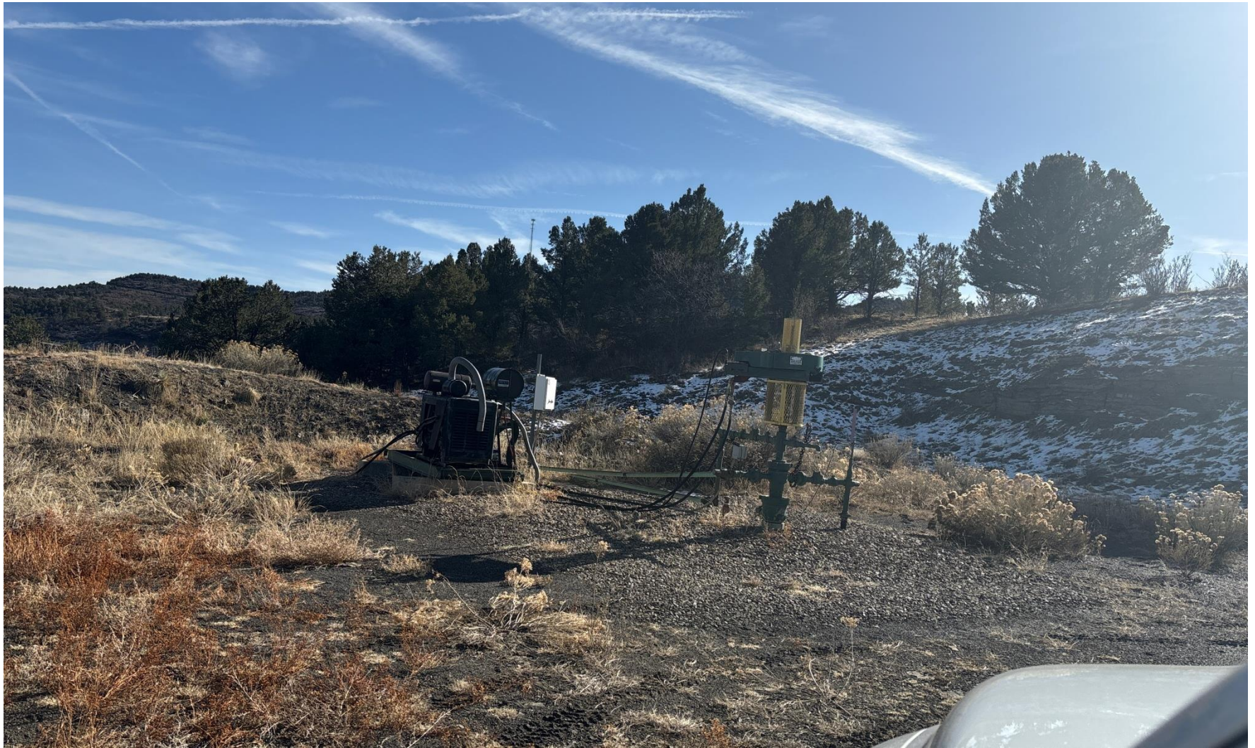
PHOTO 3: WELLHEAD AND EQUIPMENT. WEEDS NEED MAINTAINED AROUND EQUIPMENT AND LOCATION.
