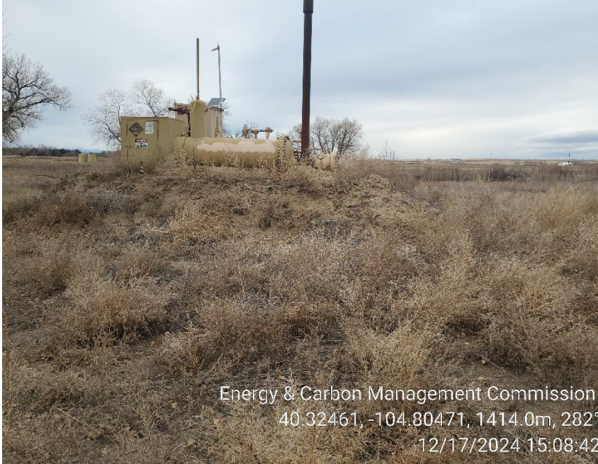
Production facility and debris
