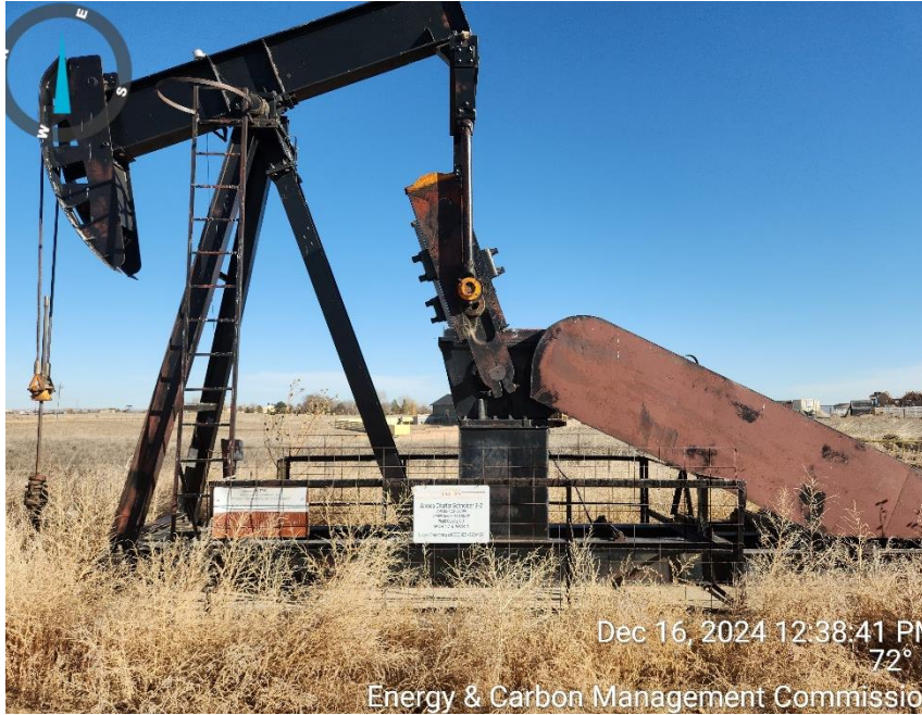
Photo 1 well head and equipment
