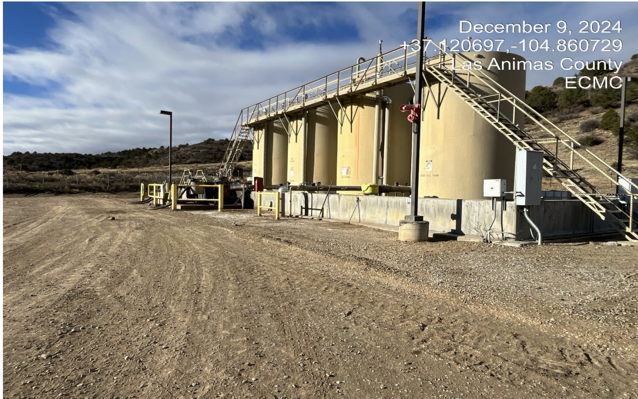
Photo 4. Facing toward the tank battery. The open top tank has been removed.
