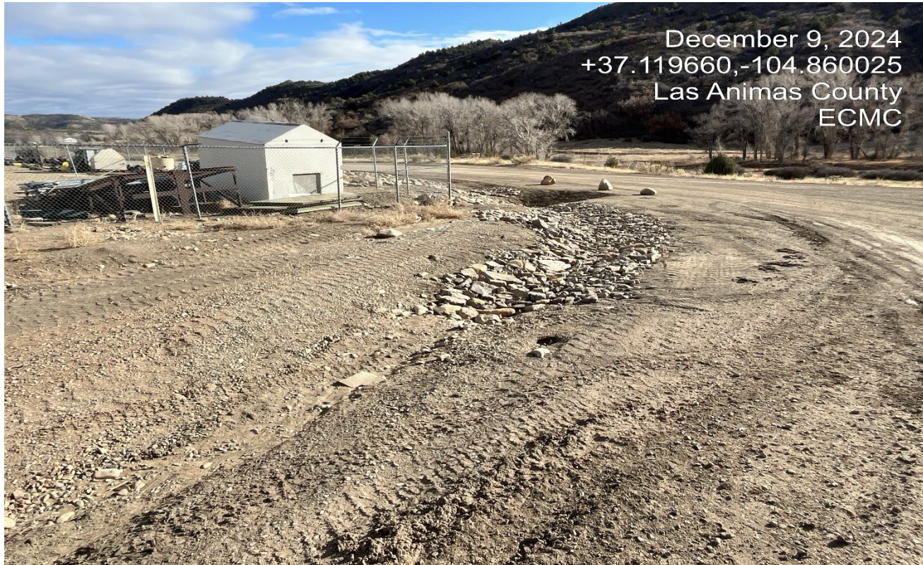
Photo 2. Facing southwest toward the access road adjacent to the main road. Additional rock rip rap has been installed to armor the roadside where erosion was occurring.
