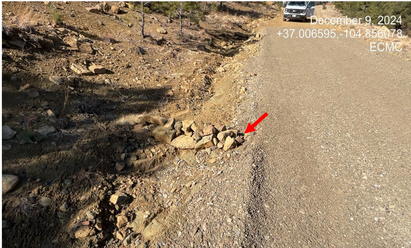
Photo 2. Facing There are some rock check dams installed but stormwater has already eroded around the out side.
