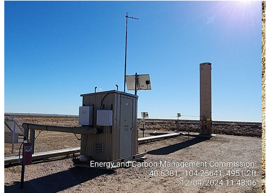
Photo 4 – Gas Meter and ECD
