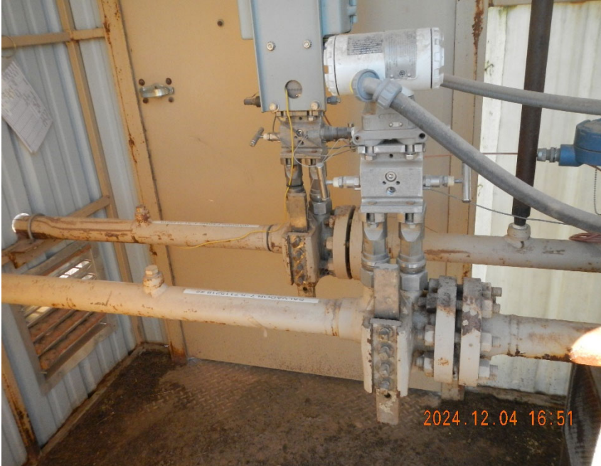
5. Gas meter inside meter shed.
