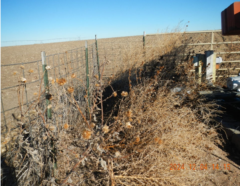
3. Dried vegetation inside wellhead fencing.
