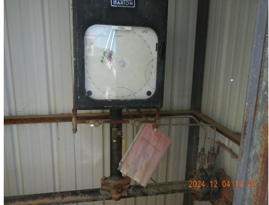
6. Shared gas meter inside shed.
