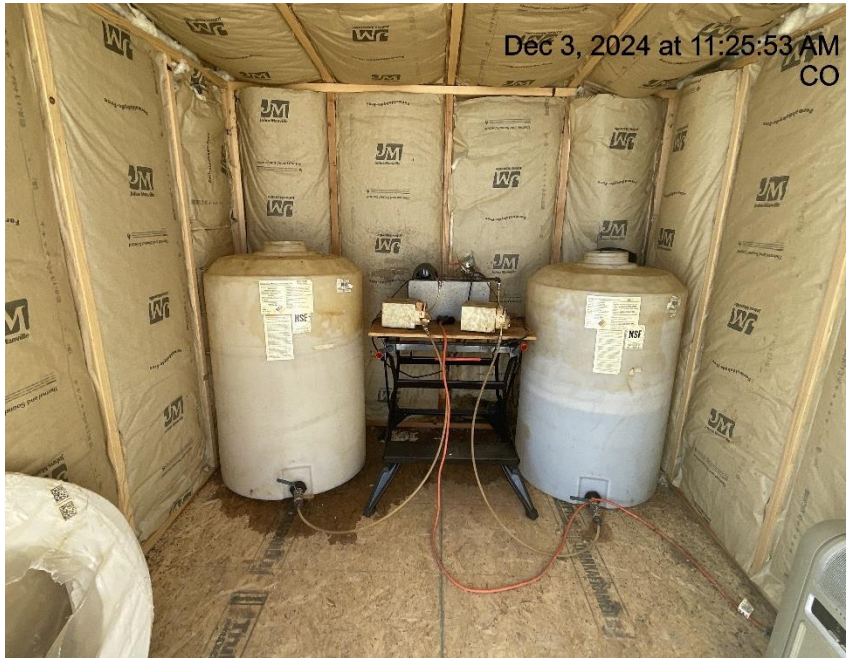
Photo # 2030 Chemical tanks located in shed, outside of shed is not labeled to indicate potential hazards inside.
