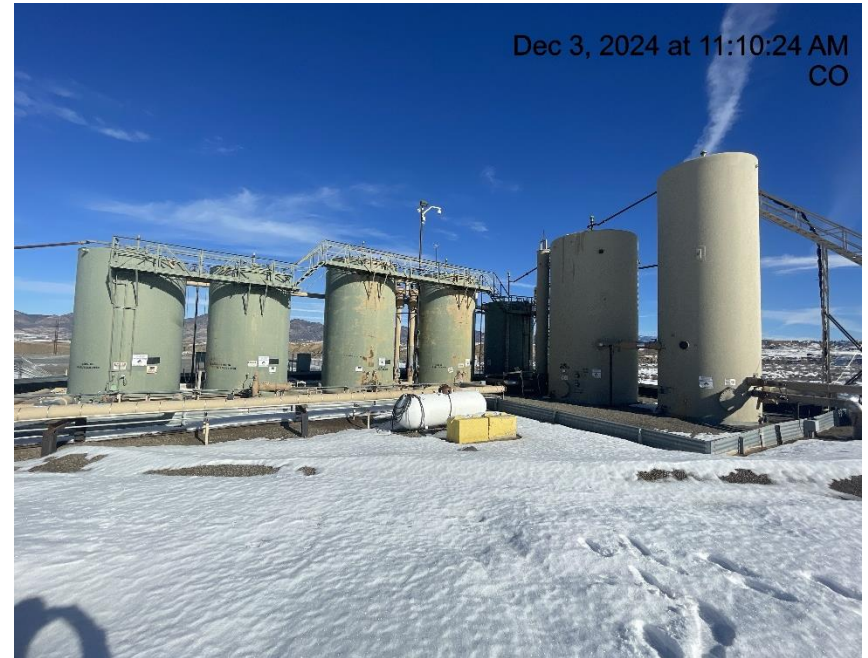
Photo # 2031 Battery lacks signage
