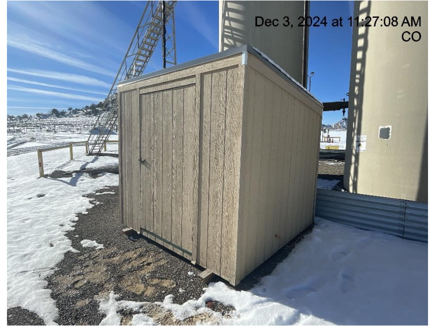
Photo # 2029 Chemical tanks located in shed, shed is not labeled to indicate potential hazards inside.
