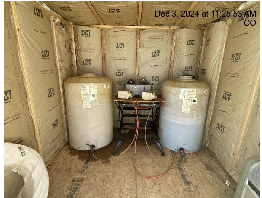
Photo # 2033 Chemical tanks in shed lack BMP's
