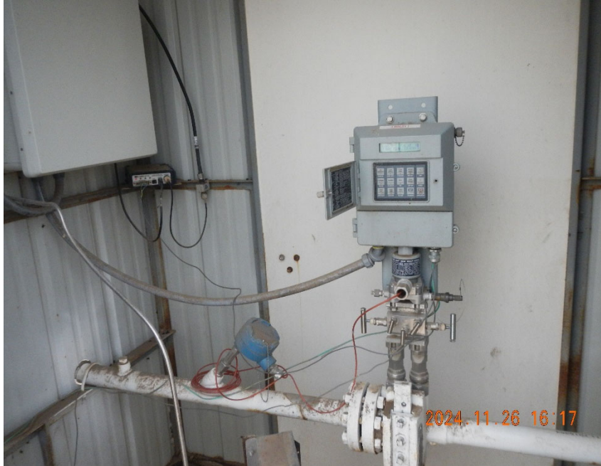
5. Gas meter inside meter shed.
