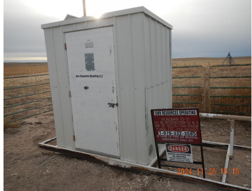
4. Well sign and meter shed at shared remote metering location.
