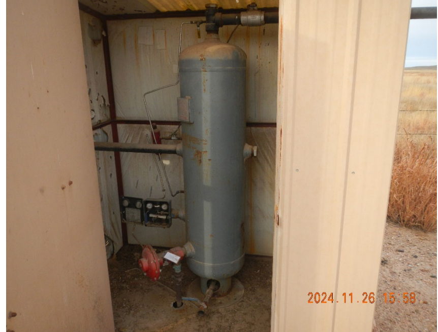
6. Vertical separator inside remote separator shed.
