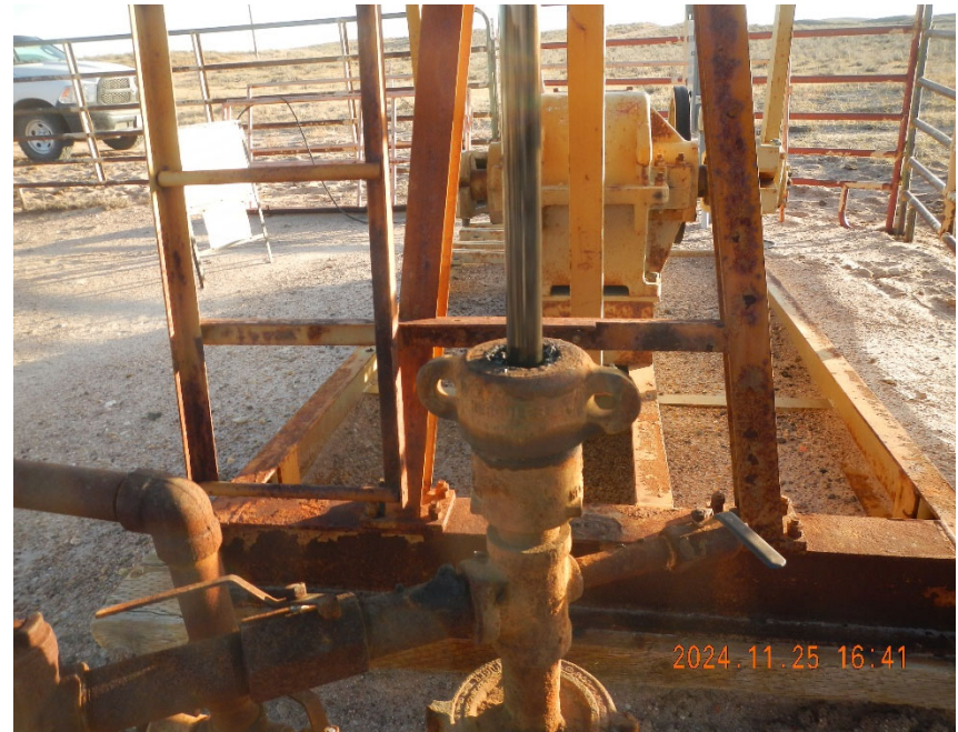
2. View of wellhead packing area.
