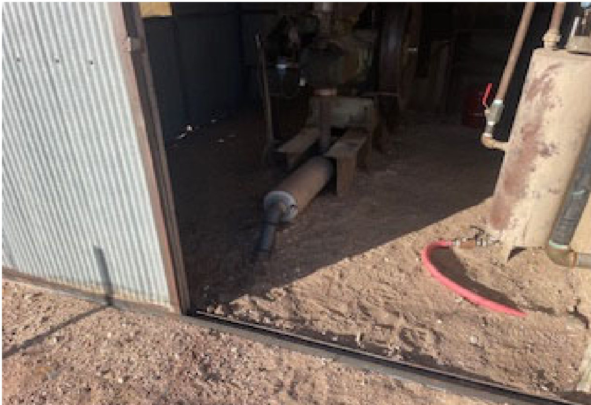
Pump Jack engine room area
