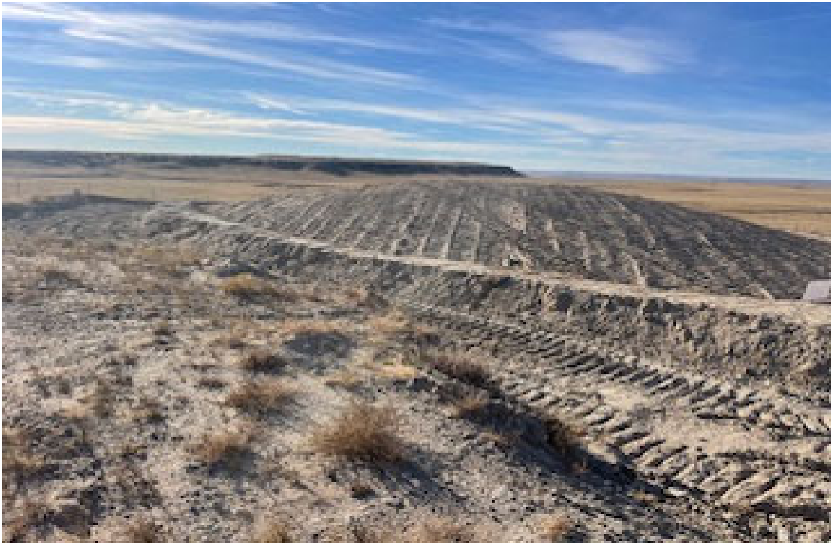
Scraped up soil from potential impacted area West of the excavation with a berm and signage
