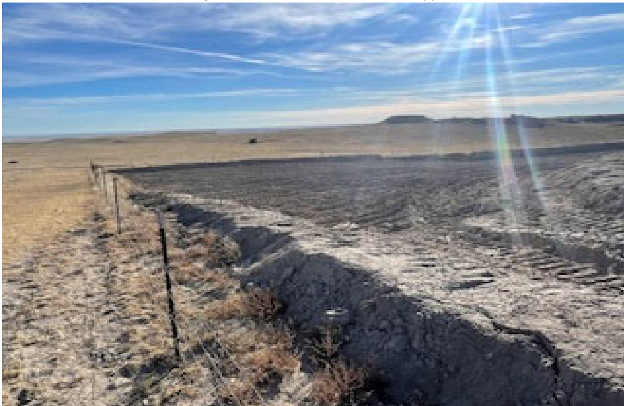
East side of excavation looking South, Weeds removed and area ripped for storm water erosion
