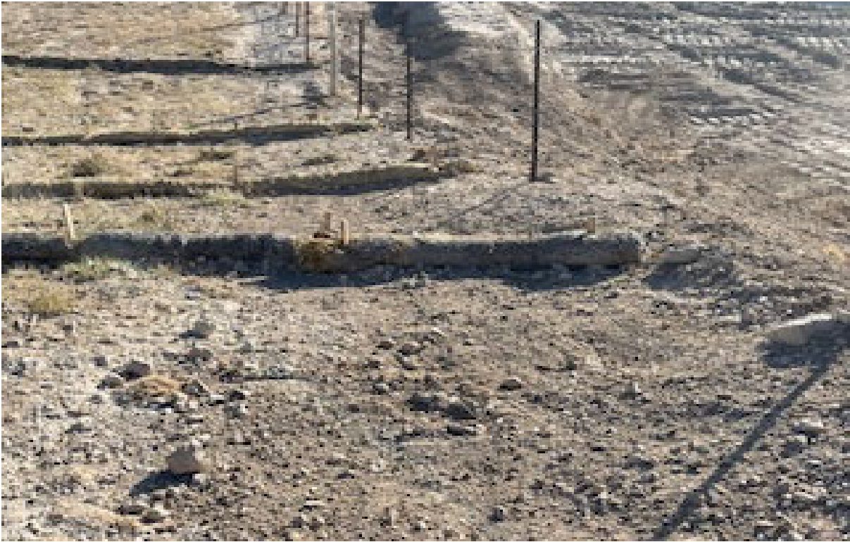
Area South of Pumping jack, Storm water erosion fixed and Straw Wattles installed, trenched and backfilled
