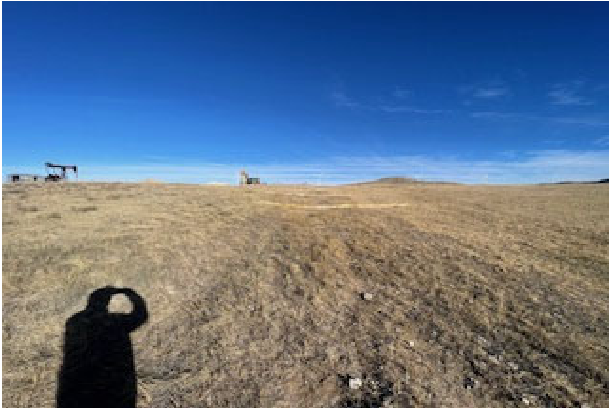
Straw Wattles installed South of old Separator Area, Standing South of wattles looking North
