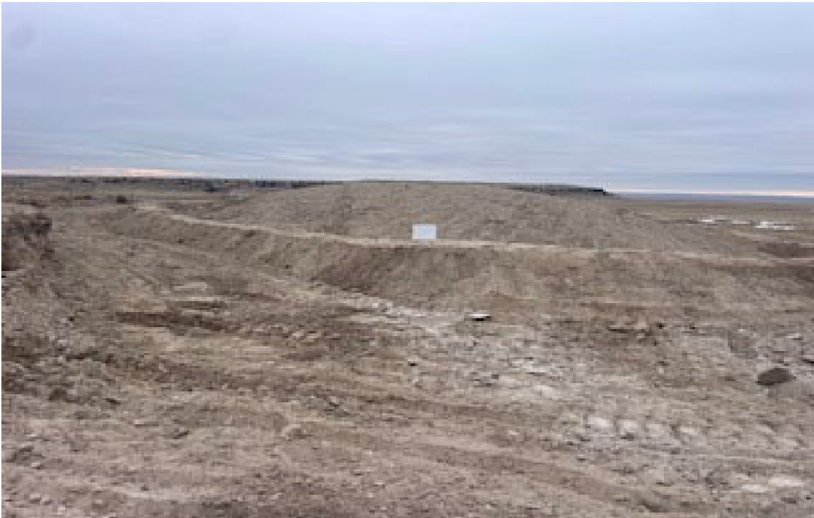
Soil scraped up from potential impacted area on South end of excavation with a berm and signage
