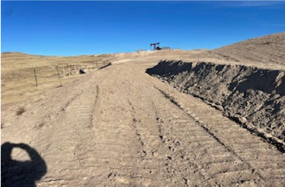
Northwest end of excavation. Perimeter berm has been improved and track packed
