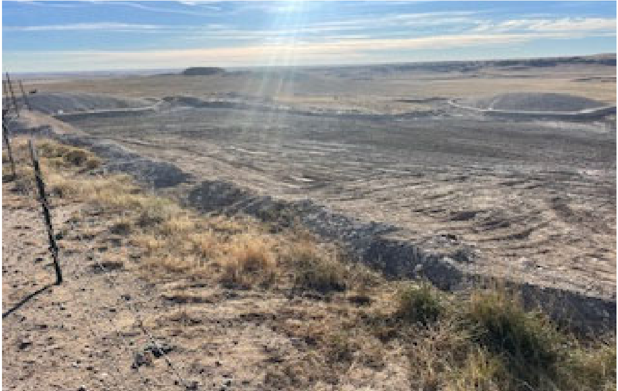
Noxious Weeds removed from excavation area and ripped for storm water erosion
