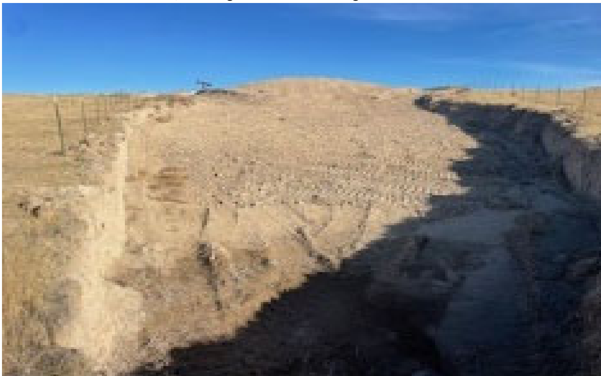
West end of excavation, standing on West end looking East. All trash and debris removed
