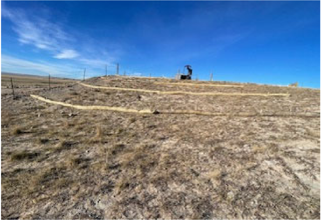
Straw Wattles installed South of Pump Jack looking from the South to the North
