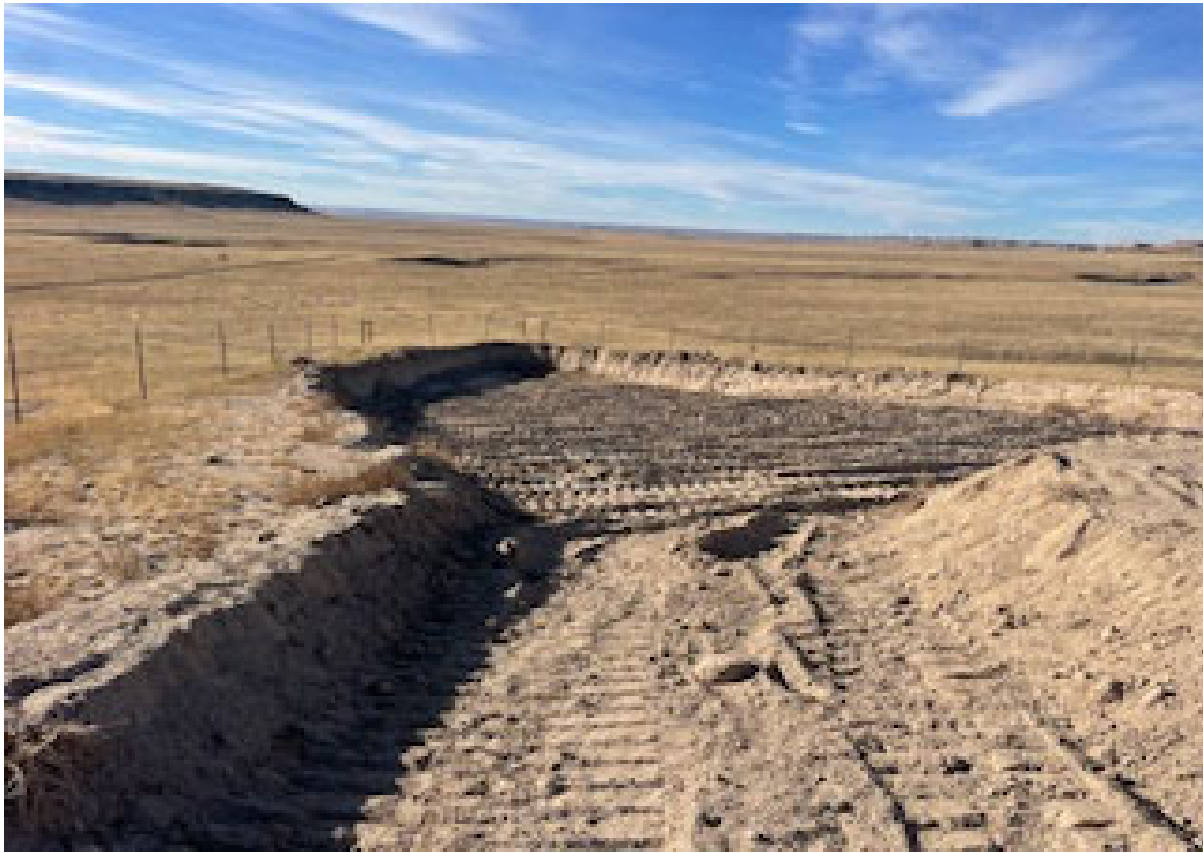
West end of excavation, weeds removed and ripped for storm water erosion
