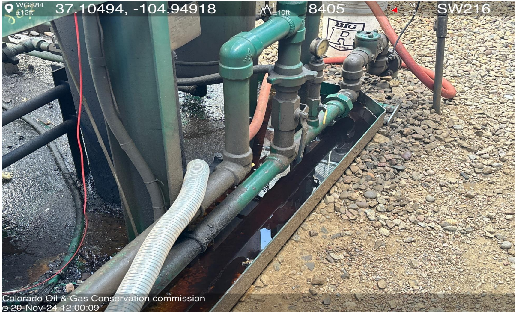
PHOTO 7: OILY WASTE FROM LEAK IN HYDRAULIC MOTOR HAS FILLED SKID AND HAS SPILLED OVER CAUSING IMPACT SOIL SURROUNDING SKID. DRAIN OILY WASTE REPAIR ALL LEAKS AND REMOVE OR TREAT IMPACTED SOIL PER RULE 1002..(2).D & 1002.f.(2)B, Comply with general provisions of the oil and gas act for wildlife protection AND SB-181. 11/21/2024.
