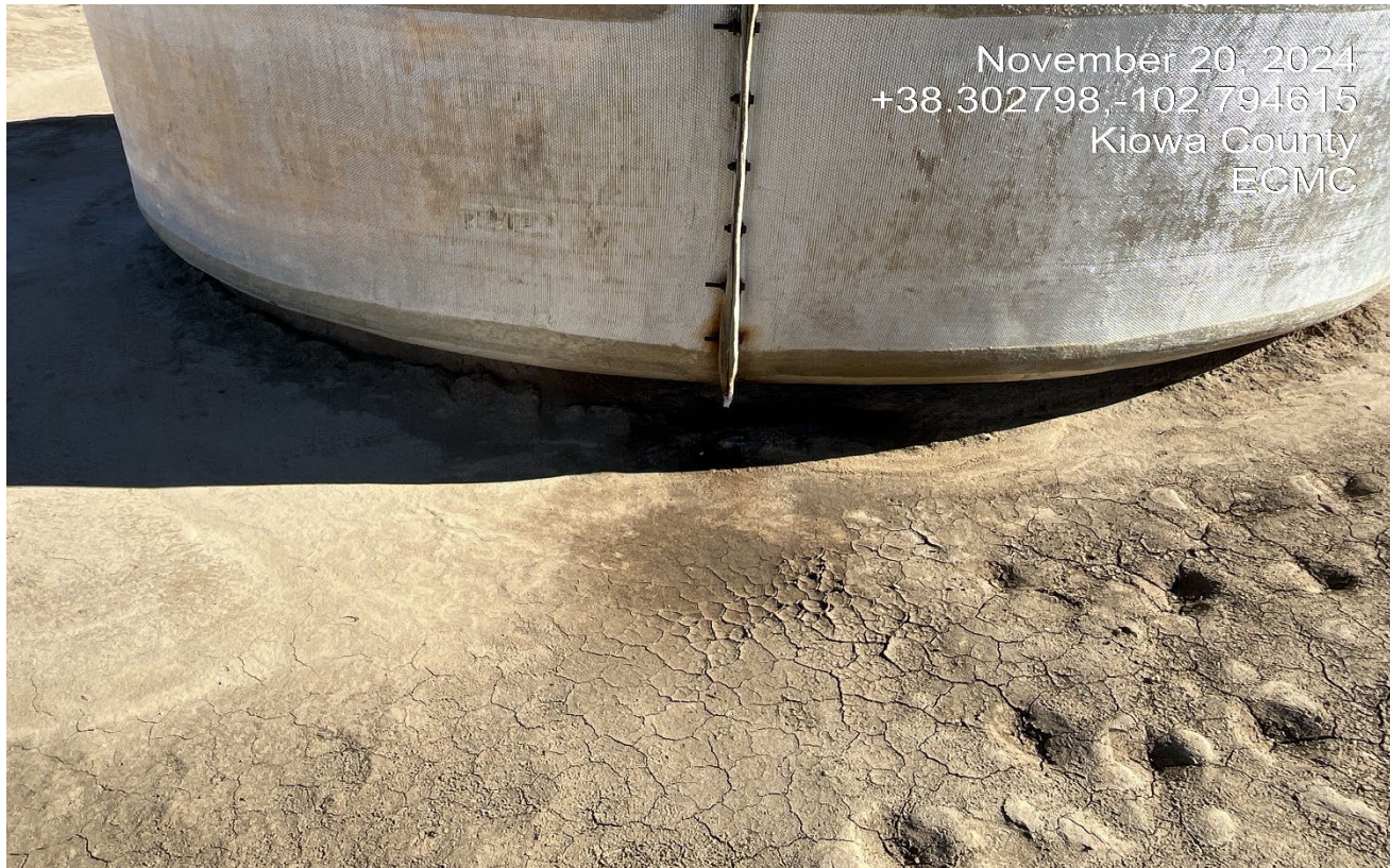
Photo 3. There is a slight leak at the tank seam.
