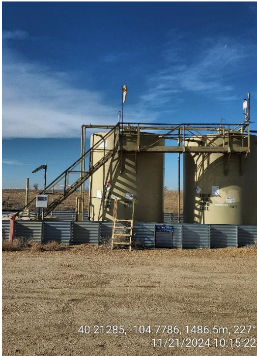
Battery West Side
