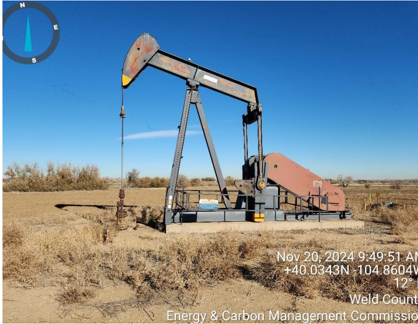
Photo 1 well head and equipment
