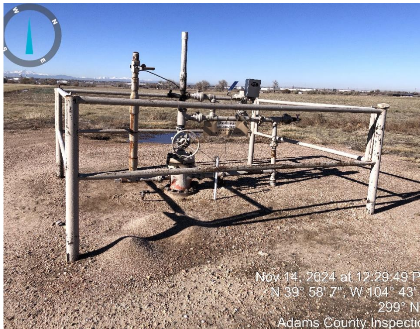
Photo #3 Well head.
