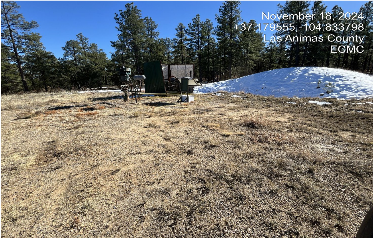
Photo 3. Facing toward the wellhead.
