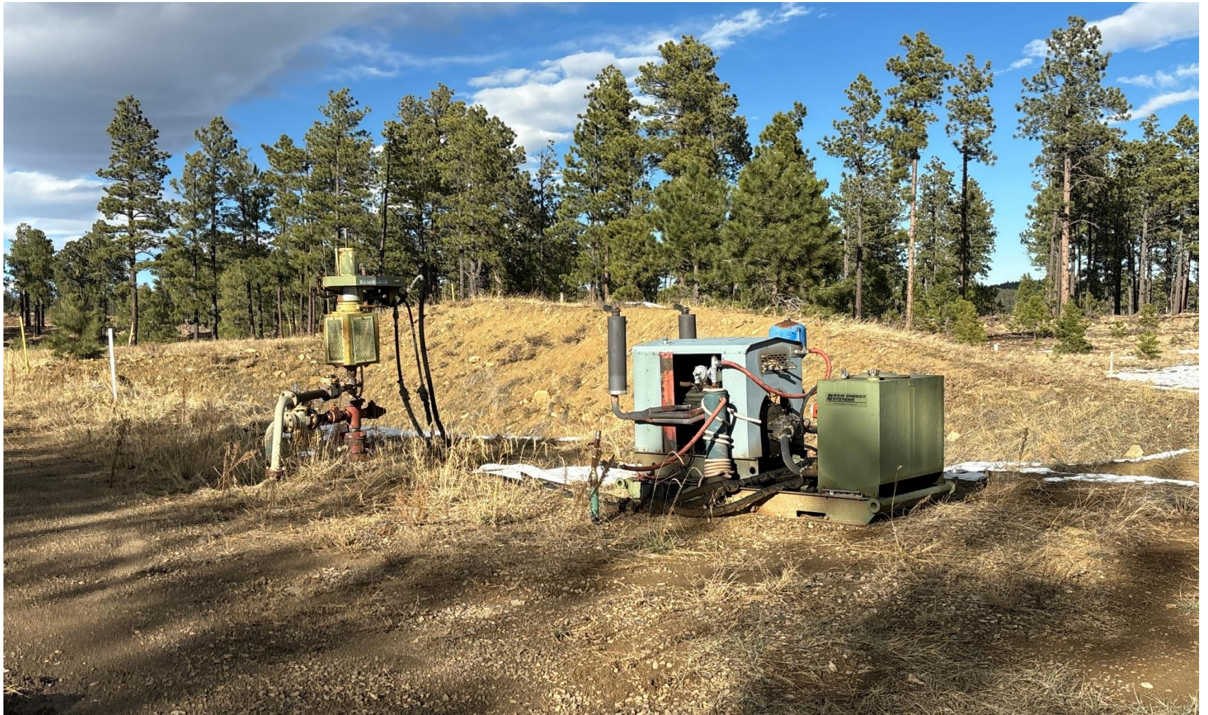
PHOTO 4: R WELLHEAD AND EQUIPMENT.
