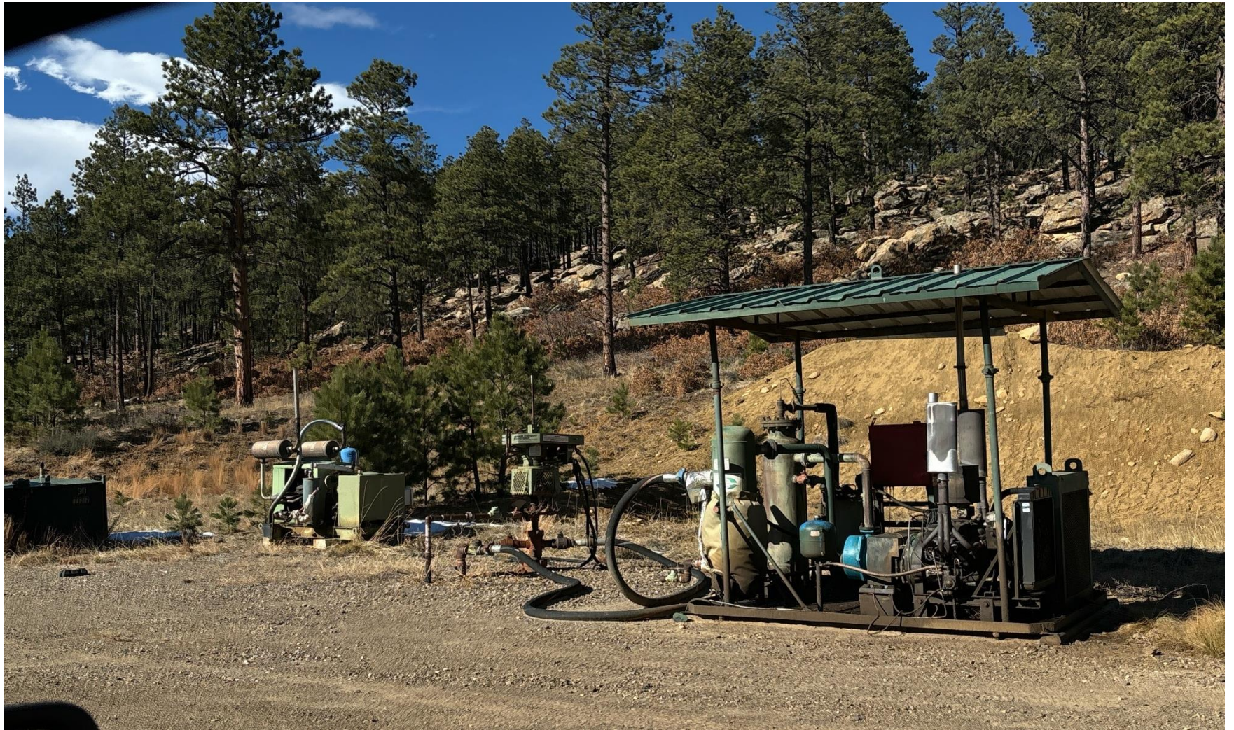
PHOTO 3: WELLHEAD AND EQUIPMENT.
