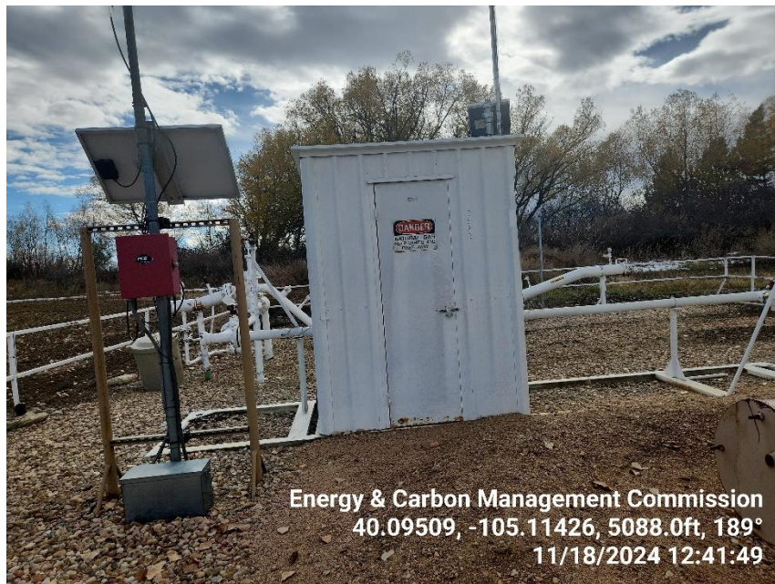
Photo 5 Gas Meter Run.
