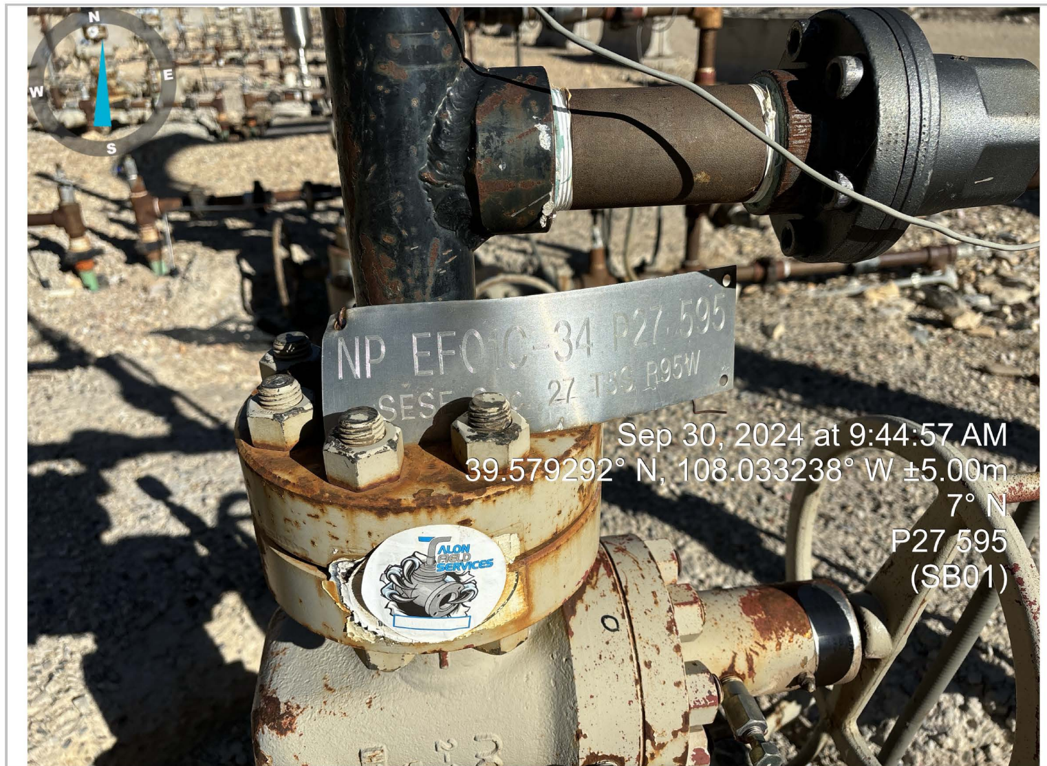
1C-34 Wellhead ID Tag
