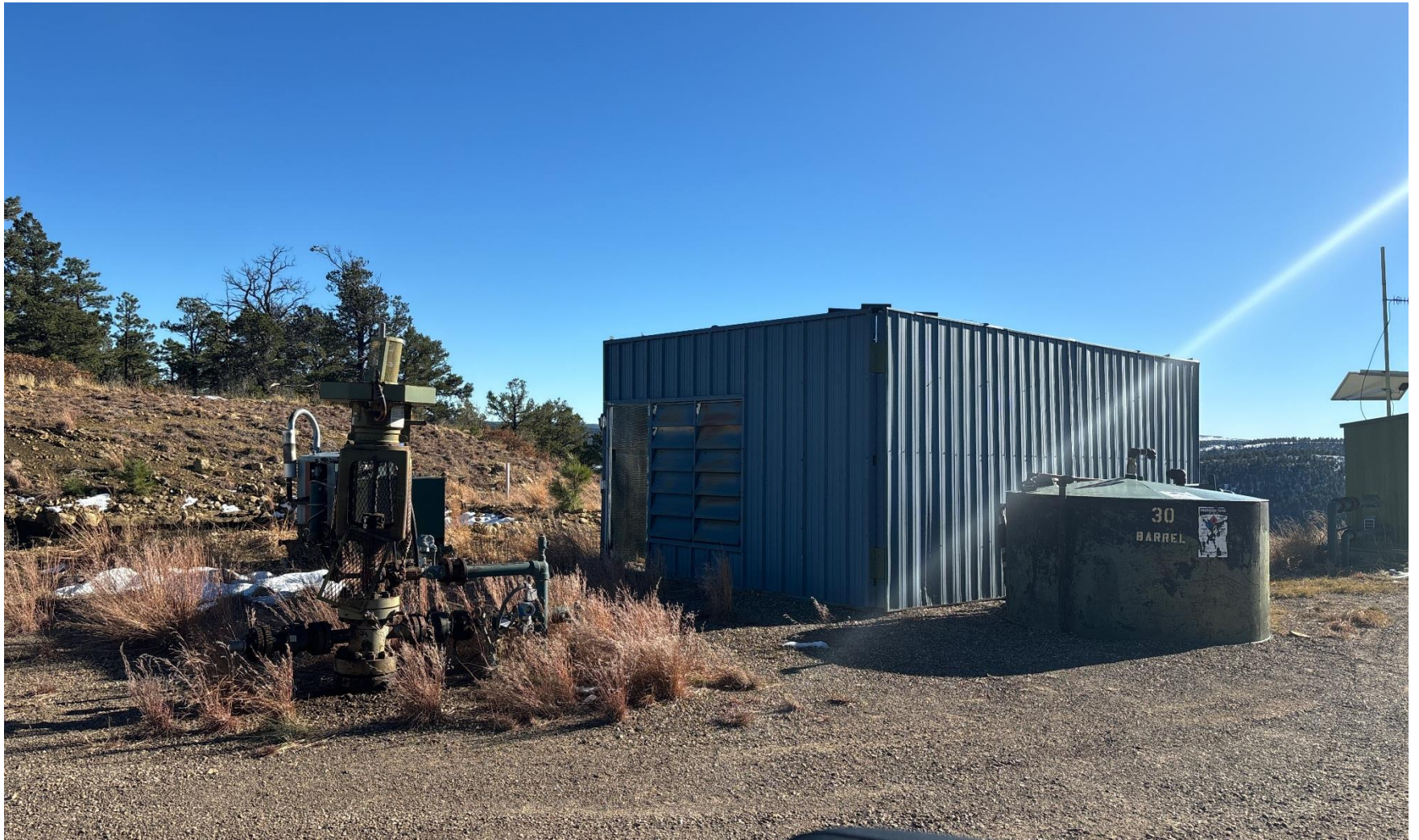
PHOTO 3: WELLHEAD AND EQUIPMENT.
