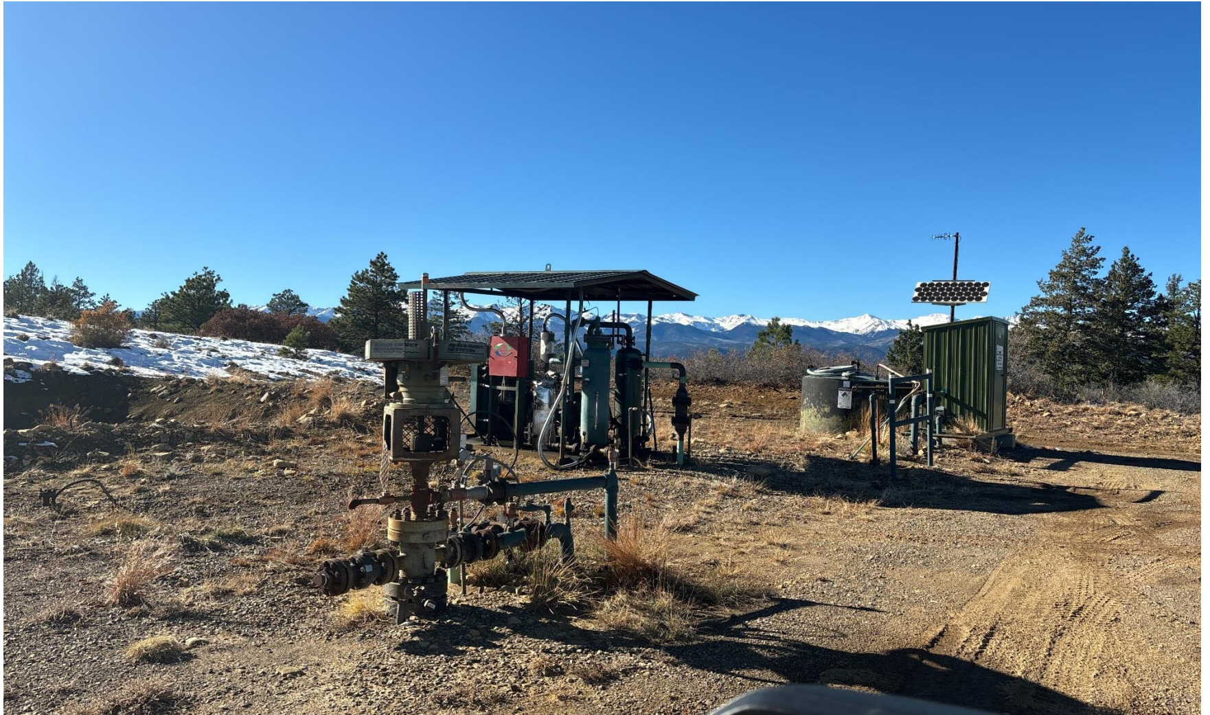
PHOTO 3: WELLHEAD AND EQUIPMENT.
