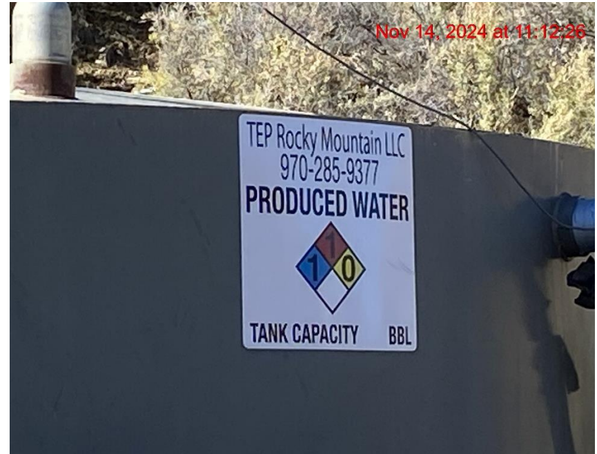
Label Does Not State Tank Capacity – Photo #04910
