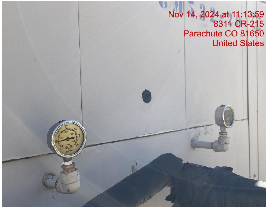
Wildlife Entry Hazard – Photo #04914
