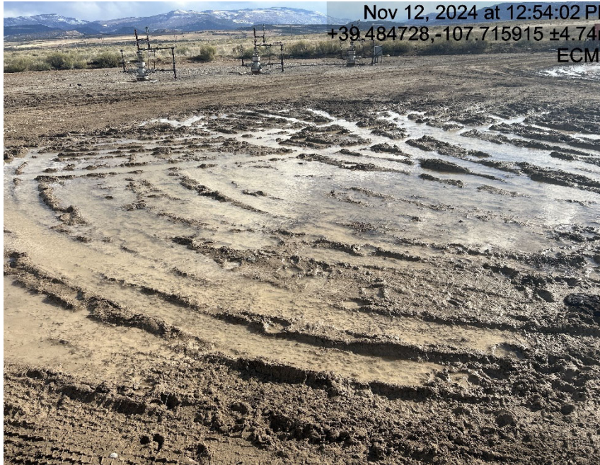
Lack of stabilization/ compaction
