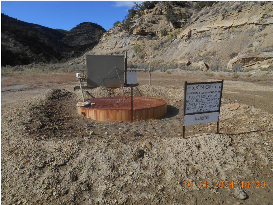
Separator and Blowdown tank
