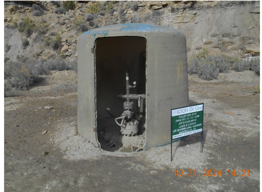
Wellhead with sign
