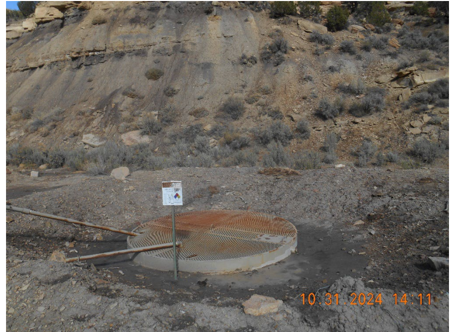
Tank Battery (Blowdown)
