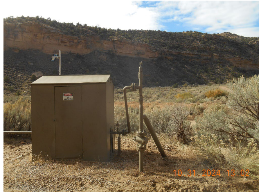
Meter housing Located ~375' due E
