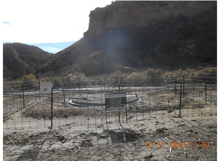
Tank Battery (Blowdown)
