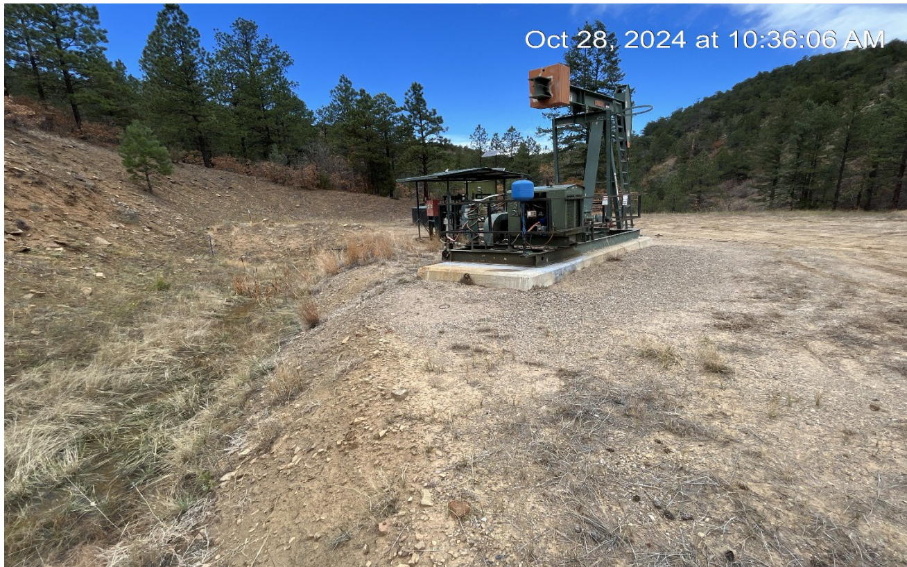
Photo 2. It appears the oil staining was cleaned up at the base of the pumpjack..
