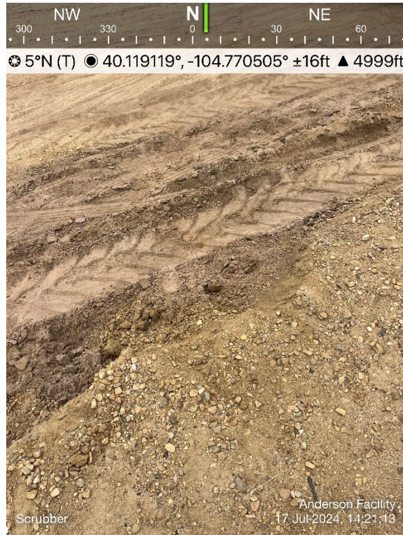
Separator Scrubber Location
