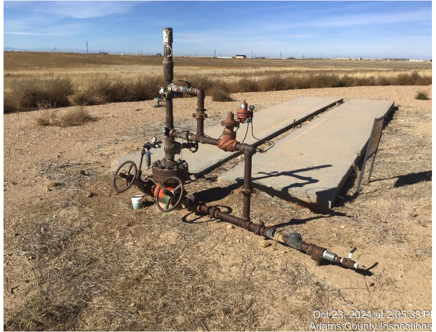
Photo #2 Well head.
