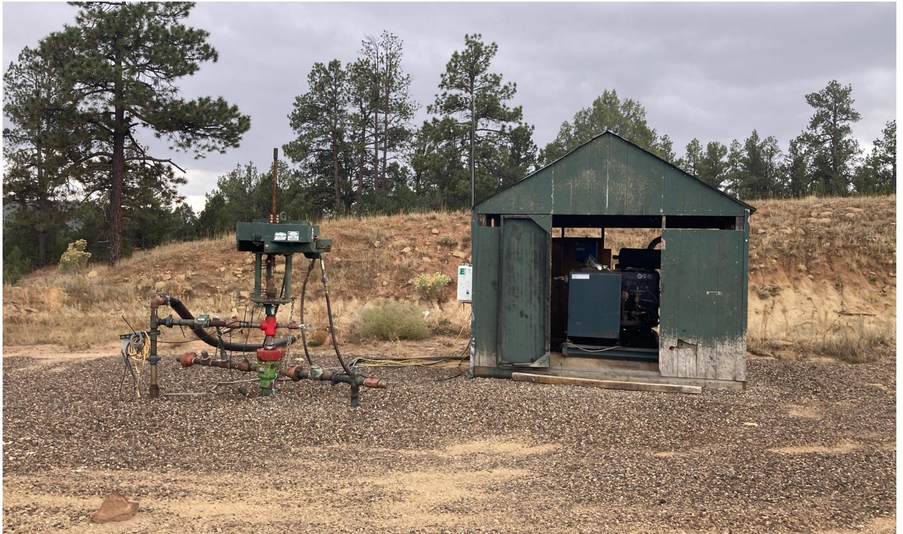
PHOTO 3: ORIG. WELLHEAD AND EQUIPMENT.
