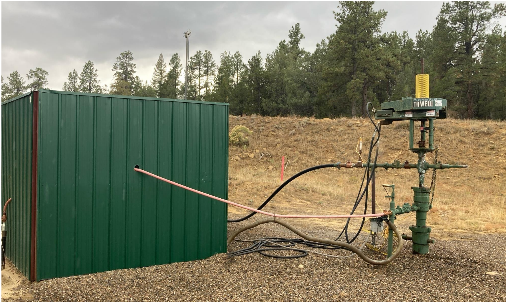
PHOTO 4: TR WELLHEAD AND EQUIPMENT.
