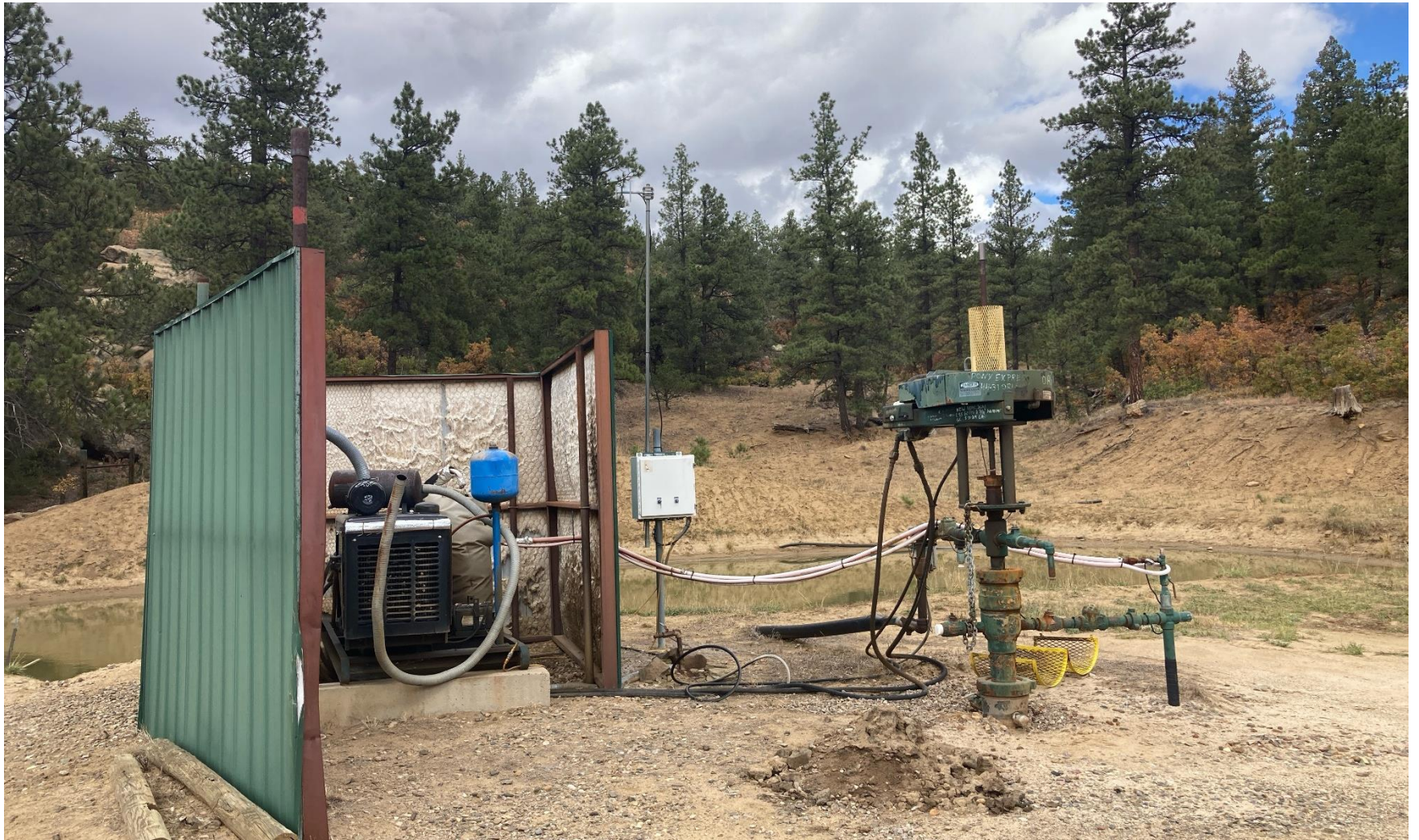
PHOTO 4: ORIG. WELLHEAD AND EQUIPMENT.
