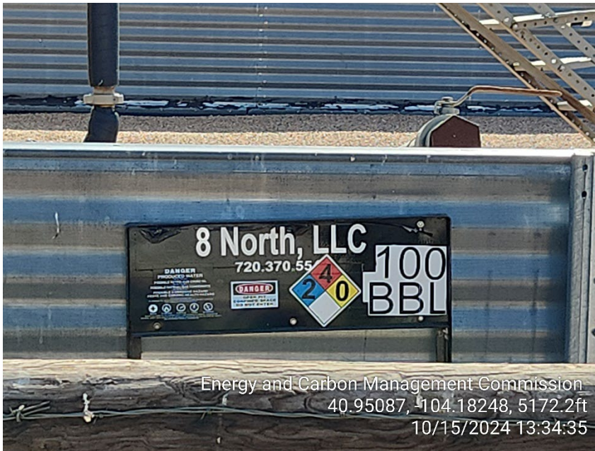
Photo 3 – New Operator Label needs installed
