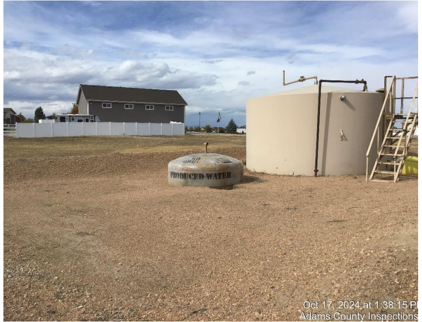
Photo #2 P/W tank.
