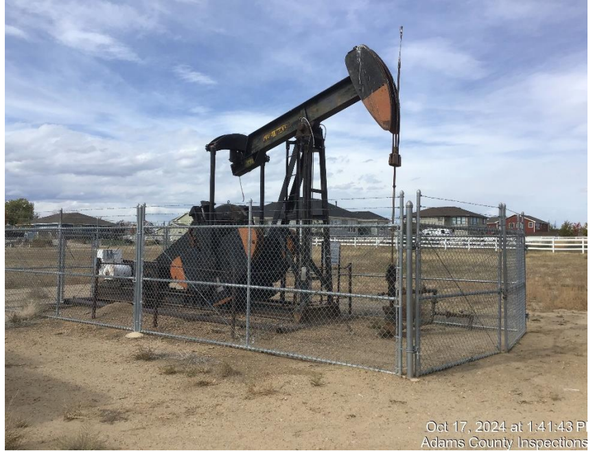
Photo #4 Pump Jack.
