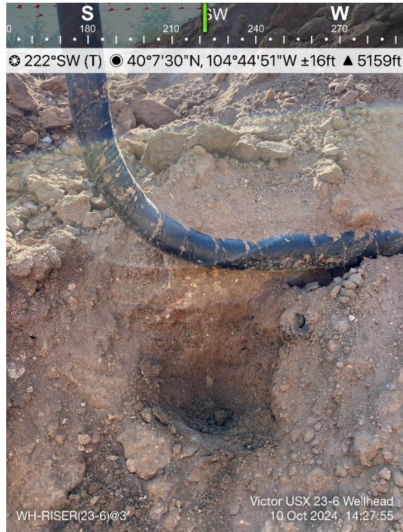
Wellhead Riser Sample Location
