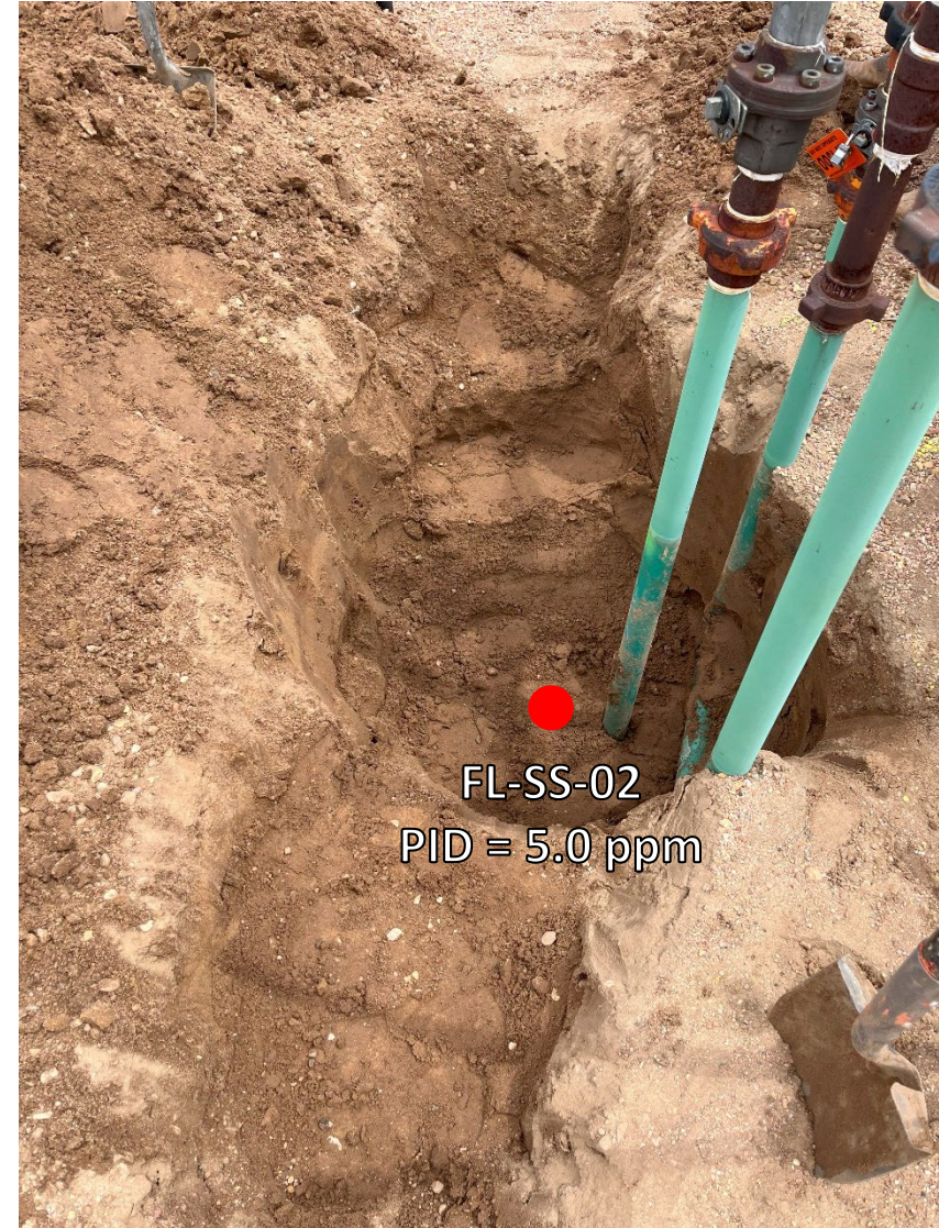
Looking west at flowline Pt B/terminus at separator
