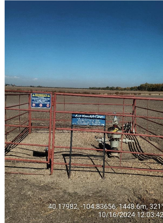
Current Inspection 05-123-24759 NISHIMOTO 23-36
