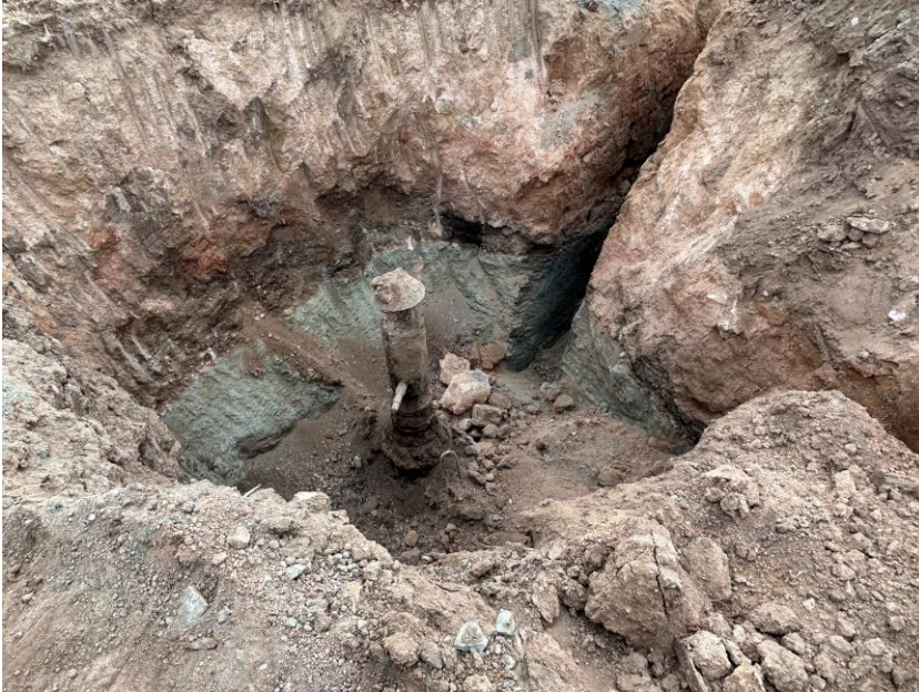
Well 20-3 Wellhead excavation looking southwest. North and west orientated trenches excavated to determine extent of petroleum contamination, (dark layer on top of weathered shale).
