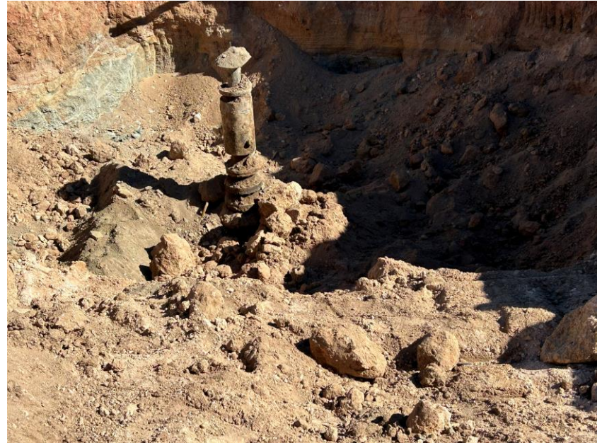
Well 20-3 Wellhead excavation looking southeast at south and east walls of excavation after removal of contaminated layer.
