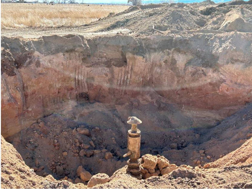
Well 20-3 Wellhead excavation looking southwest at south and west walls of excavation after removal of contaminated layer.
