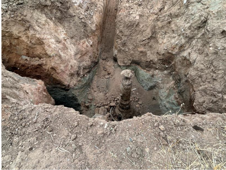
Well 20-3 Wellhead excavation looking north. North and west orientated trenches excavated to determine extent of petroleum contamination, (dark layer on top of weathered shale).
